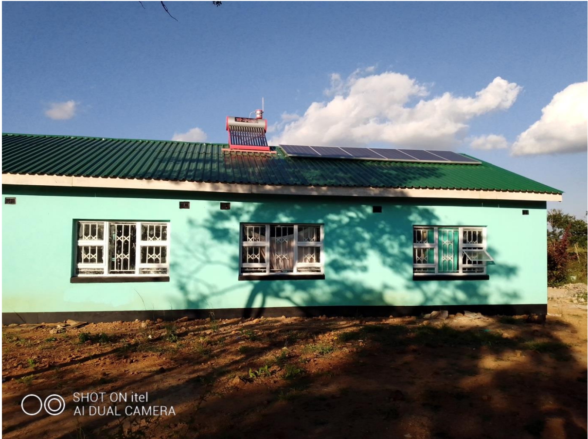
A solar geyser was installed successfully on top of the hostel
